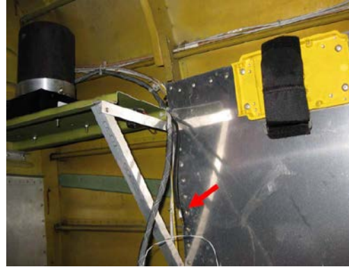
Disconnected antenna due to beacon ejection
